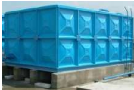
Gambar 9 Roof Water Tank
