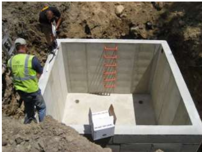
Gambar 8 Ground Water Tank
